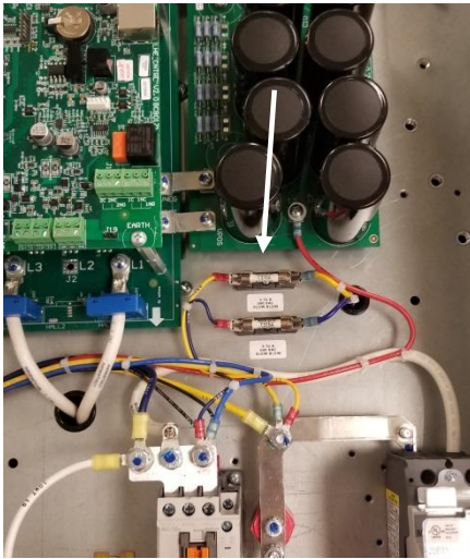
Fuses FS10 and F11 are located on the panel near the circuit breaker.
