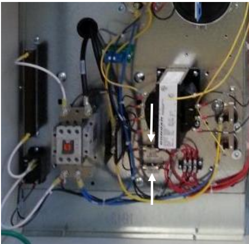
Fuses FS10 and F11 are located on the panel near the control transformer
