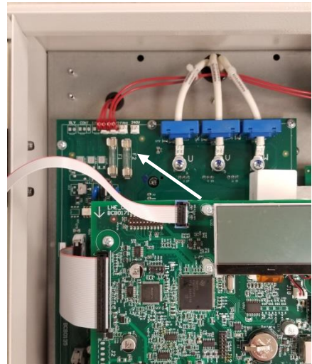
Fuses F1 and F2 are located on the circuit board beneath the display.
