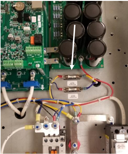
Fuses FS10 and F11 are located on the panel near the circuit breaker.
